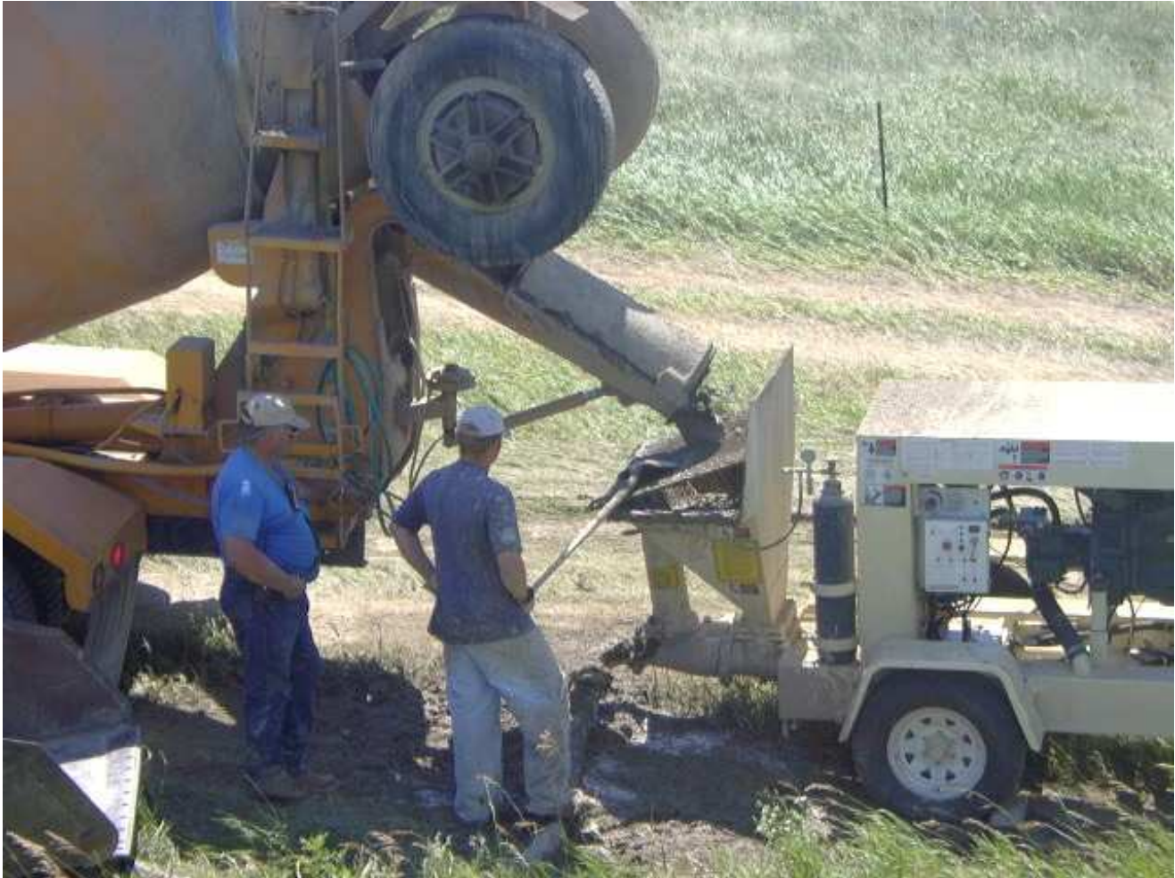
Photo 2: Grout injection in the right of way of US Highway 200. Grout was dumped from cement trucks into a grout pump and pumped into underground mined workings.
