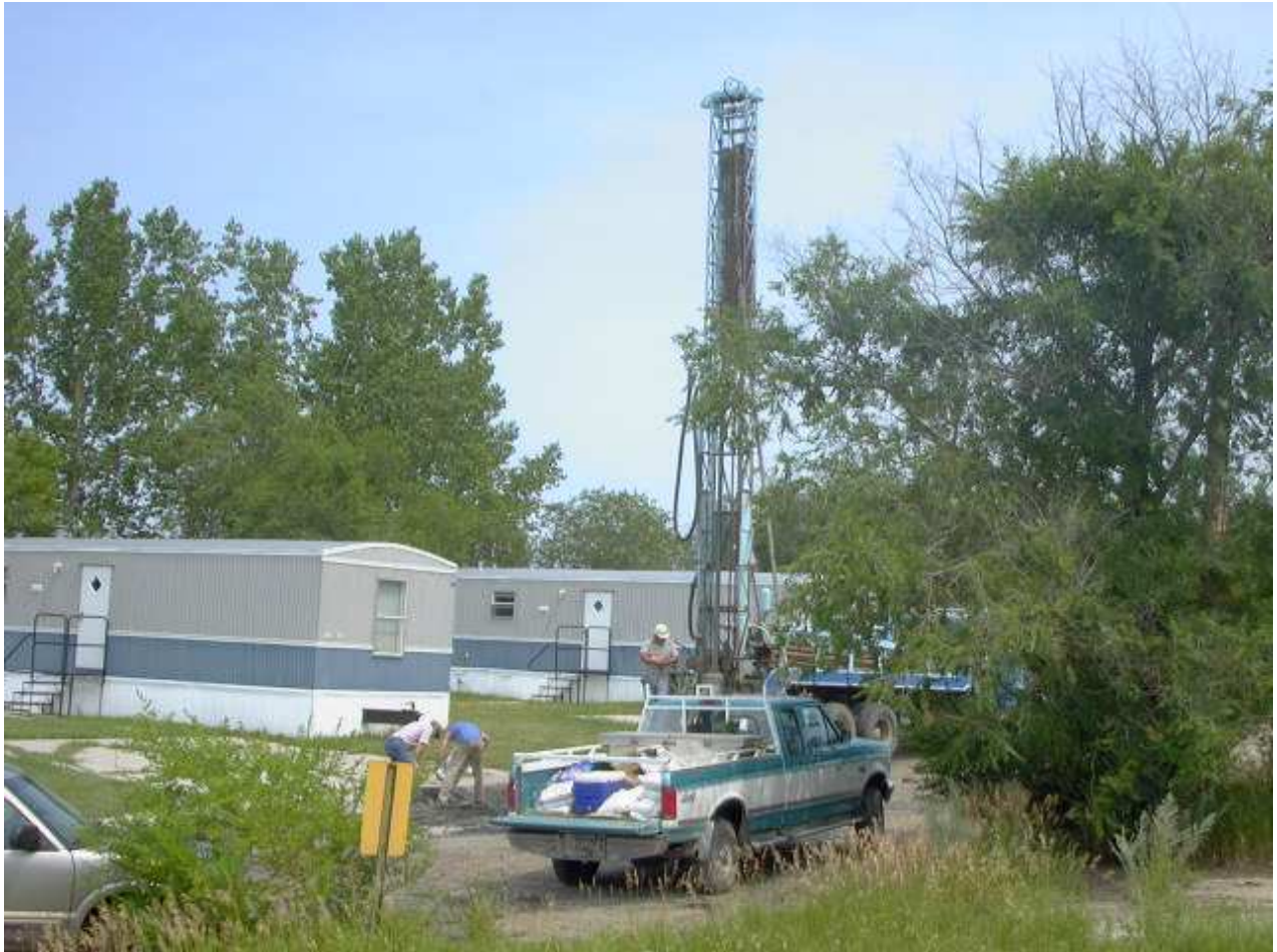
Photo 3: Drilling at Sun Valley Court in Beulah. Grout injection was conducted at this area in a 1992 project. Confirmation drilling and limited grout injection was conducted in 2003.
