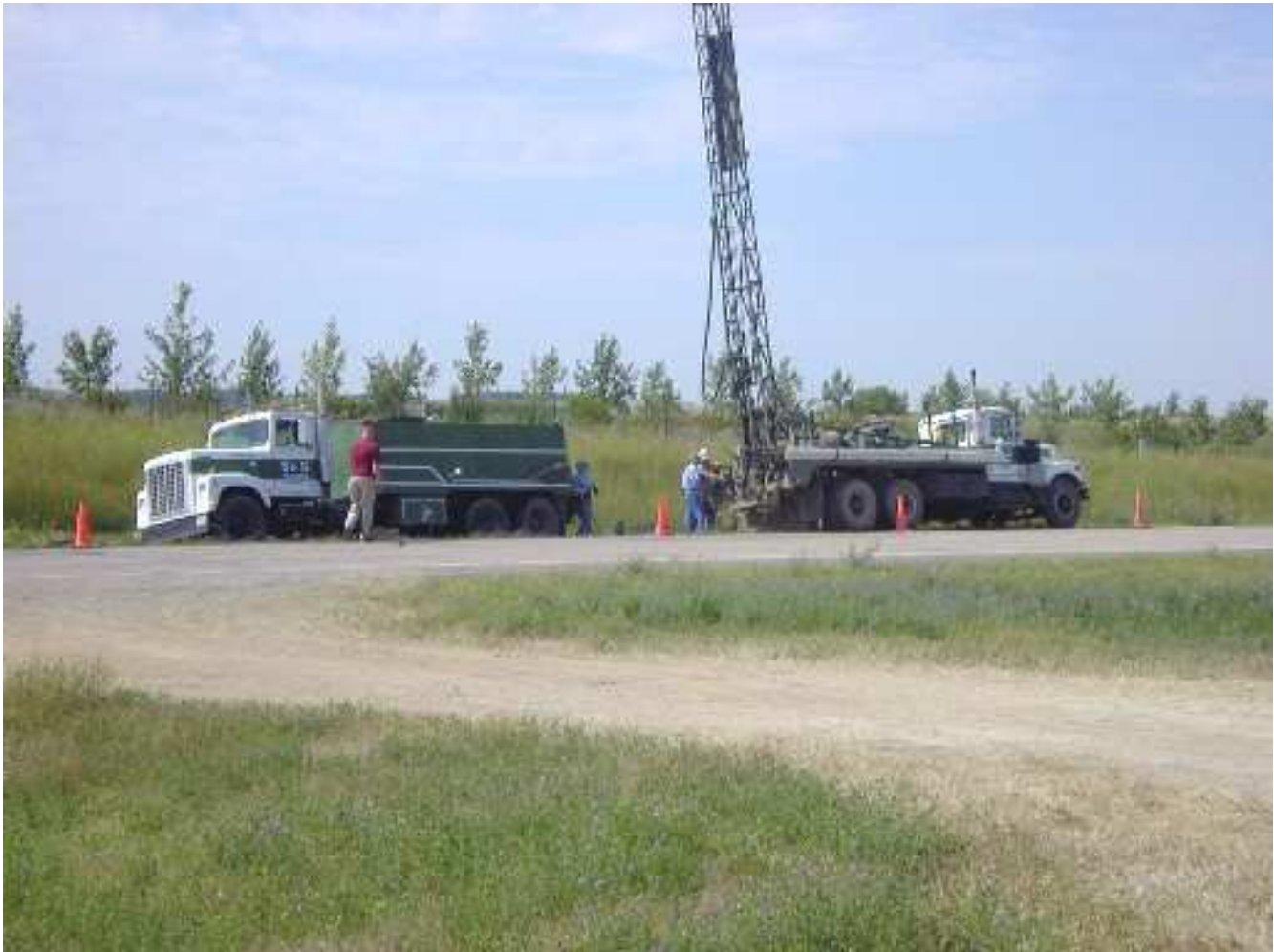
Photo 1: Drilling at Buechler Site. Drilling and grout injection were conducted along an undermined segment of ND Highway 23 about eight miles south of the city of Sawyer.
