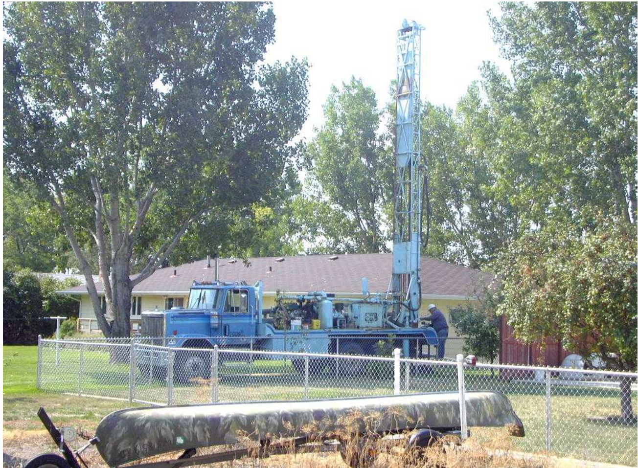
Photo 2: Exploratory/Geophysical Drilling, Garrison Site. Exploratory and geophysical drilling was conducted at two residential sites in and near Garrison, ND. This drilling revealed underground mined workings and additional reclamation is planned for these areas in 2004.
