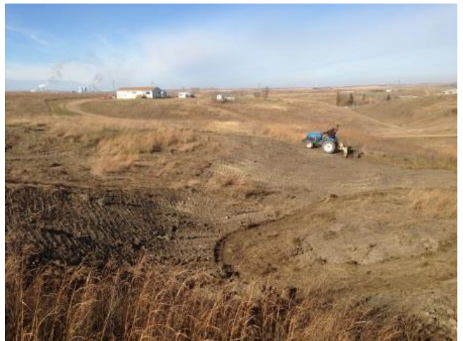
Tilling and seeding was done after all sinkholes were filled and topsoil was replaced. Eight sinkholes were filled on Mike's property and the cost was about $2350.
