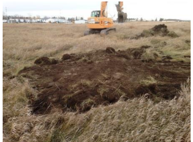
This shows a sinkhole after topsoil was replaced. The excavator is moving to compact and add topsoil to another. Twenty-four sinkholes were filled at Garrison at the cost of $6970.
