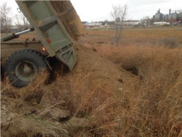
Sinkhole filling was conducted at Garrison November 4-6, 2015. Fill dirt was taken from a nearby sand pit.
