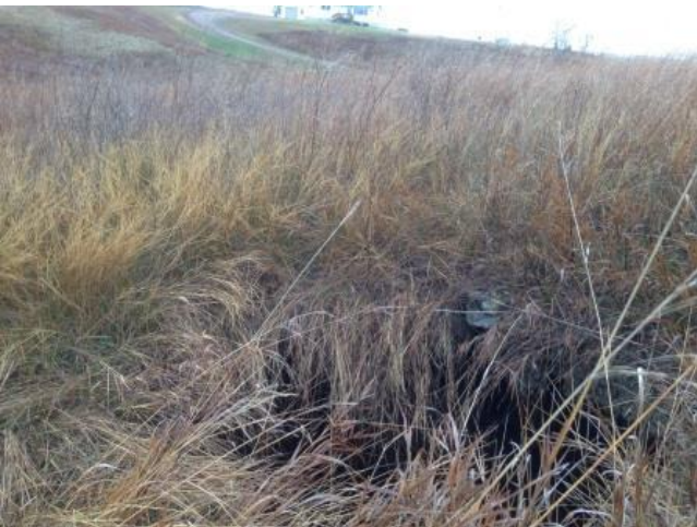
This shows a sinkhole on property owned by Mike Eslinger, north of Beulah. It was about 8 feet in diameter below the surface and 10 feet deep. It was very dangerous because it was difficult to see until you were right on top of it.
