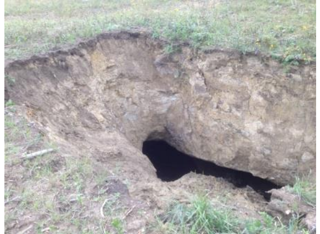
This is a close-up of the sinkhole at the terminus of the erosion features. It was about 25 feet long, 18 feet wide and 22 feet deep.
