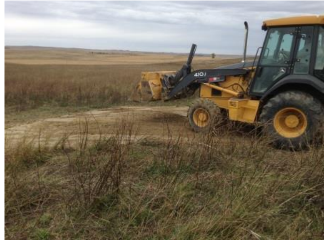
This shows one of the sinkholes at the Haynes site after it was filled but before seeding. Seven sinkholes were filled at the Haynes site and the approximate cost was $3320.
