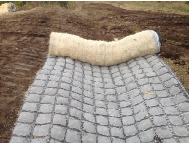
The waterway was seeded and lined with Flexamat, a tied concrete block mat used to control erosion. Vegetation can grow between the blocks and completely cover the entire mat.
