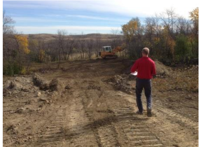
This picture shows the site after the sinkhole was filled and the erosion repaired. A waterway was constructed to contain runoff and minimize erosion.
