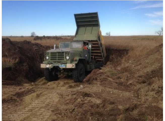
It took about 370 truckloads of dirt to fill all the sinkholes on Garner's property between October 21 and 31. The cost was $26,950.
