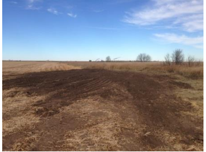
This shows the same area after the sinkhole was filled. It took about 15 truckloads of dirt to fill.
