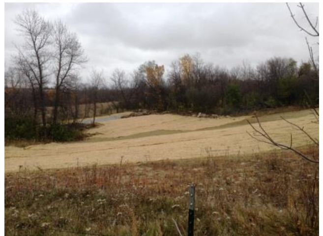
This shows the area on October 16th after all work was completed. Work at this site included filling nine sinkholes, construction of a lined waterway, and stabilizing a larger area with erosion control blankets. The cost of this work was $18,977.
