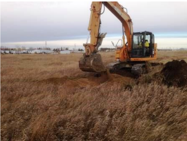
This shows an excavator compacting fill dirt in the sinkhole. Sakakawea RV is in the background and a couple sinkholes were within 20 feet of one of the RV pads.
