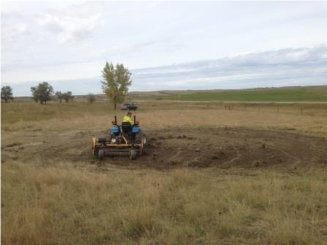
After the sinkhole was filled with nine truckloads of dirt, topsoil was replaced and the area was seeded and tilled.
