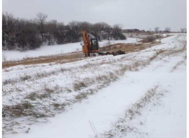
Sinkhole filling began at the Wilton Site on November 6, 2014. This shows the excavation of a sinkhole on property owned by Robert Bailey in the NE1/4 of Section 6, T142, R79, 3 miles east of Wilton.
