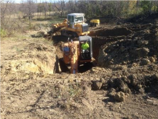
Work began at this site on October 9, 2014. The excavator had to ramp into the hole in order to completely excavate it.
