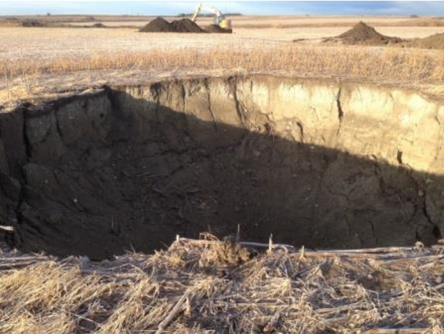
This is another of the sinkholes that were filled on Garner's property. It was about 32 feet in diameter and 12 feet deep.
