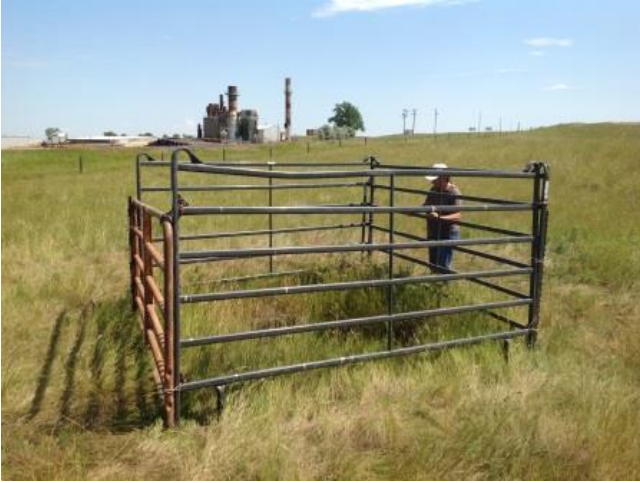
This sinkhole was reported July 1, 2014, by property owner Mike Wolf. He placed gate panels around it to keep livestock out. It was about 13 feet in diameter and 13 feet deep.
