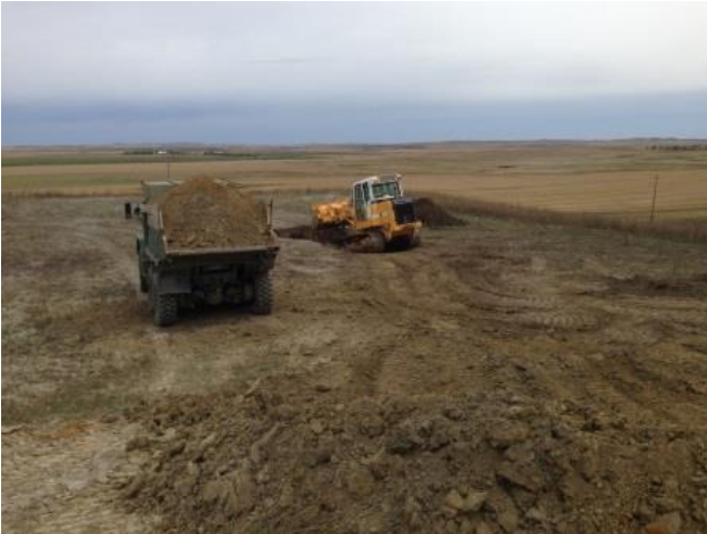
This shows the filling of a sinkhole at the Haynes Site on October 6, 2014. This hole required about 7 truckloads of dirt.
