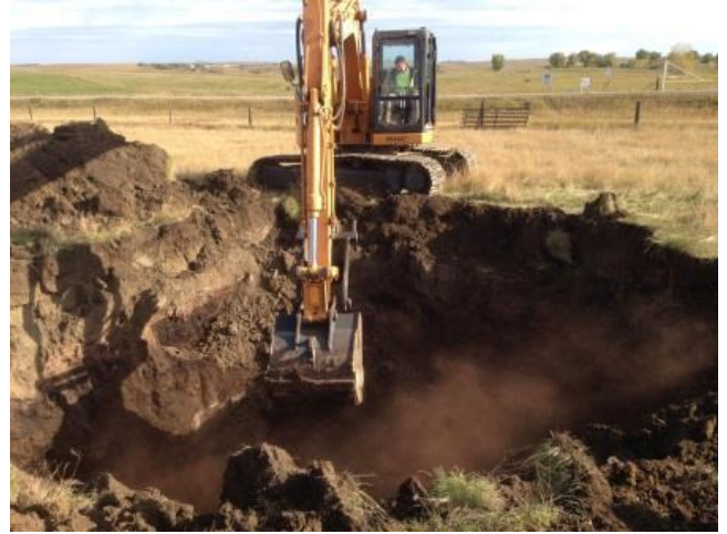
This photo was taken October 8, 2014 while the sinkhole was being excavated. Topsoil was removed and piled beside the hole.
