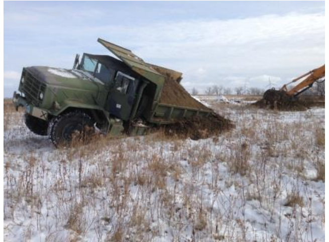
The contractor removed most of the soil from the truck with an excavator and pulled it out of the hole.
