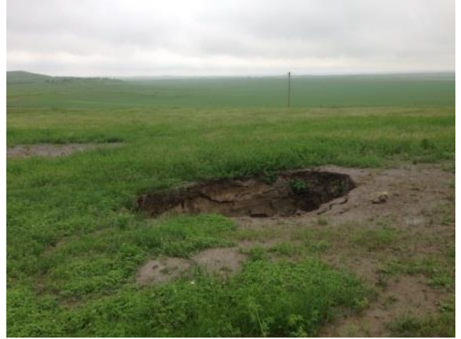
Several of the sinkholes at Haynes were very near where sinkholes had been filled in 2013.
