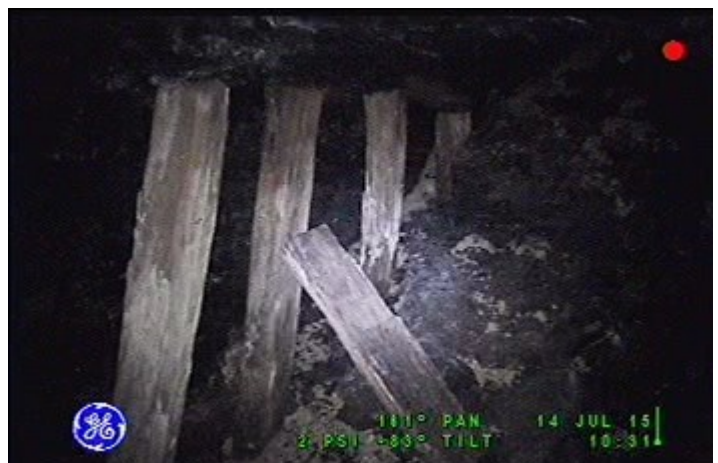
Halleck Mine: Timbers are part of the haul tunnel leading to the rooms. On the right the tunnel has partially collapsed.
