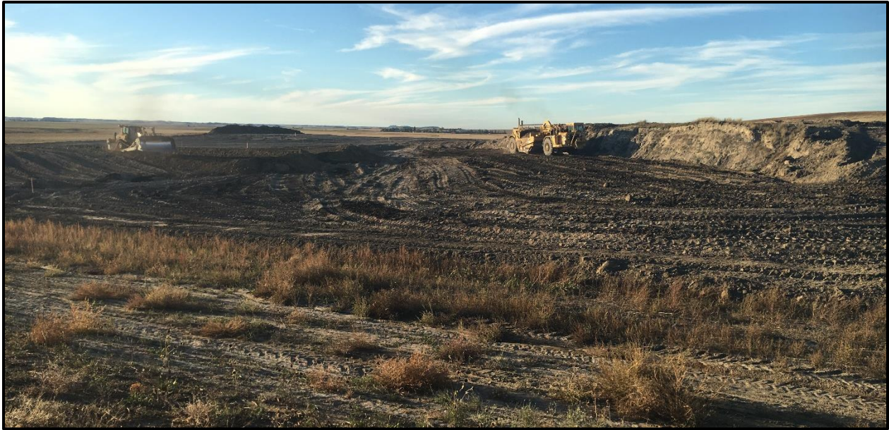
Top: Cat D8T dozer and Cat 627G scraper leveling the highwall on the north site
