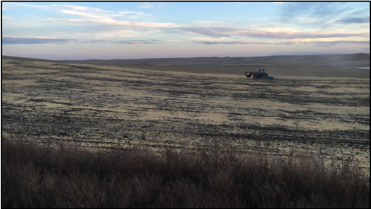
Bottom: Final grade of the south site during the process of crimping the placed straw mulch
