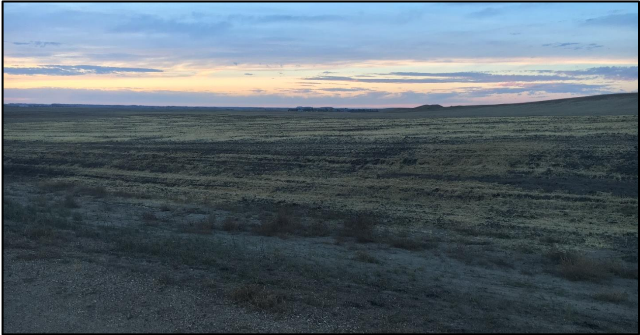
Top: Final grade of the north site after straw mulching and crimping
