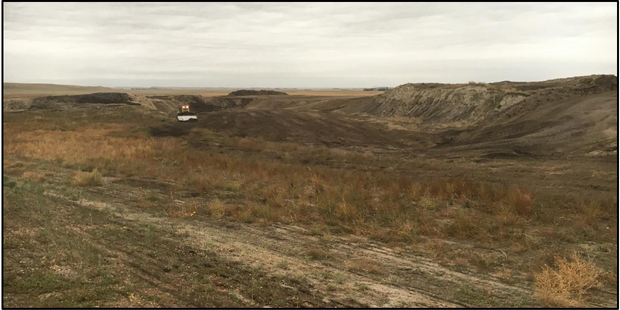
Top: Cat D8T dozer performing the topsoil stripping of the pit of the north site.
