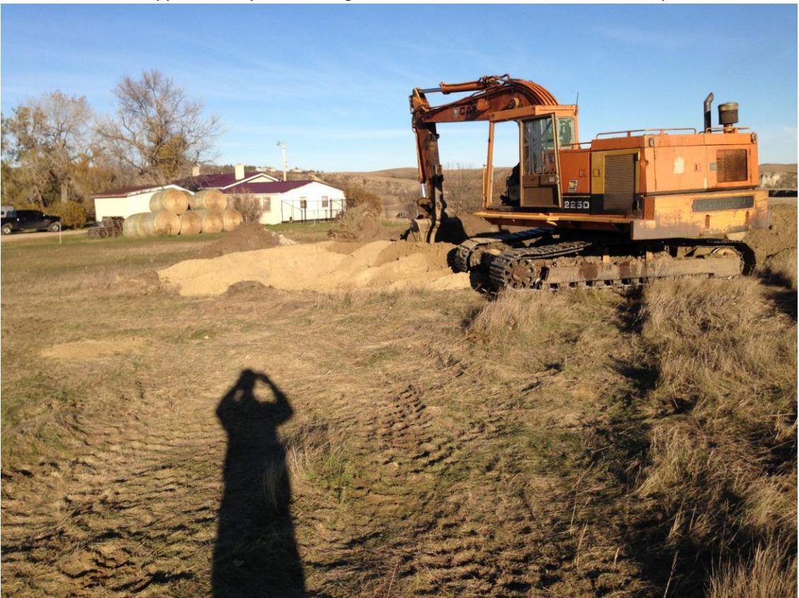
This shows the same hole when it was nearly full with 17 truckloads of dirt. Lexi's home is in the background. Eight sinkholes were filled at four properties near Dickinson on November 1–2. The cost for this work was $3703.
