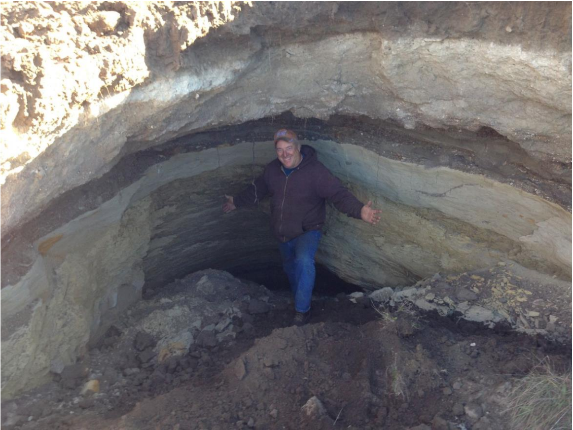
This shows contractor, Ross Smith, standing in a sinkhole on a pasture rented by Lexi Sebastian about two miles east of Dickinson. This sinkhole was approximately 33 feet long, 12 feet wide and more than 7 feet deep.
