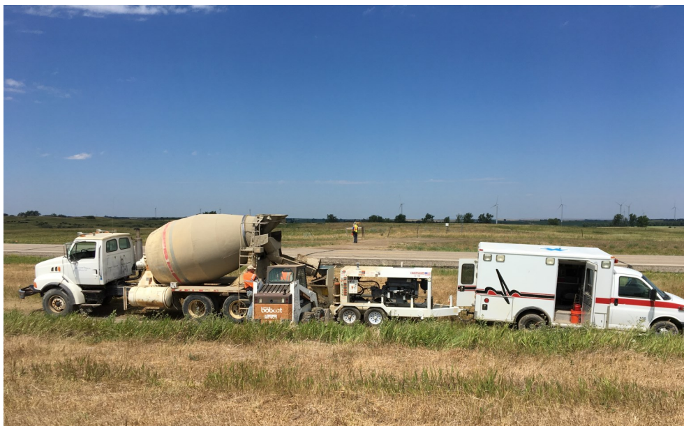
Grout Pumping in the south ditch of ND State Highway 36 about 5 miles east of Wilton.
