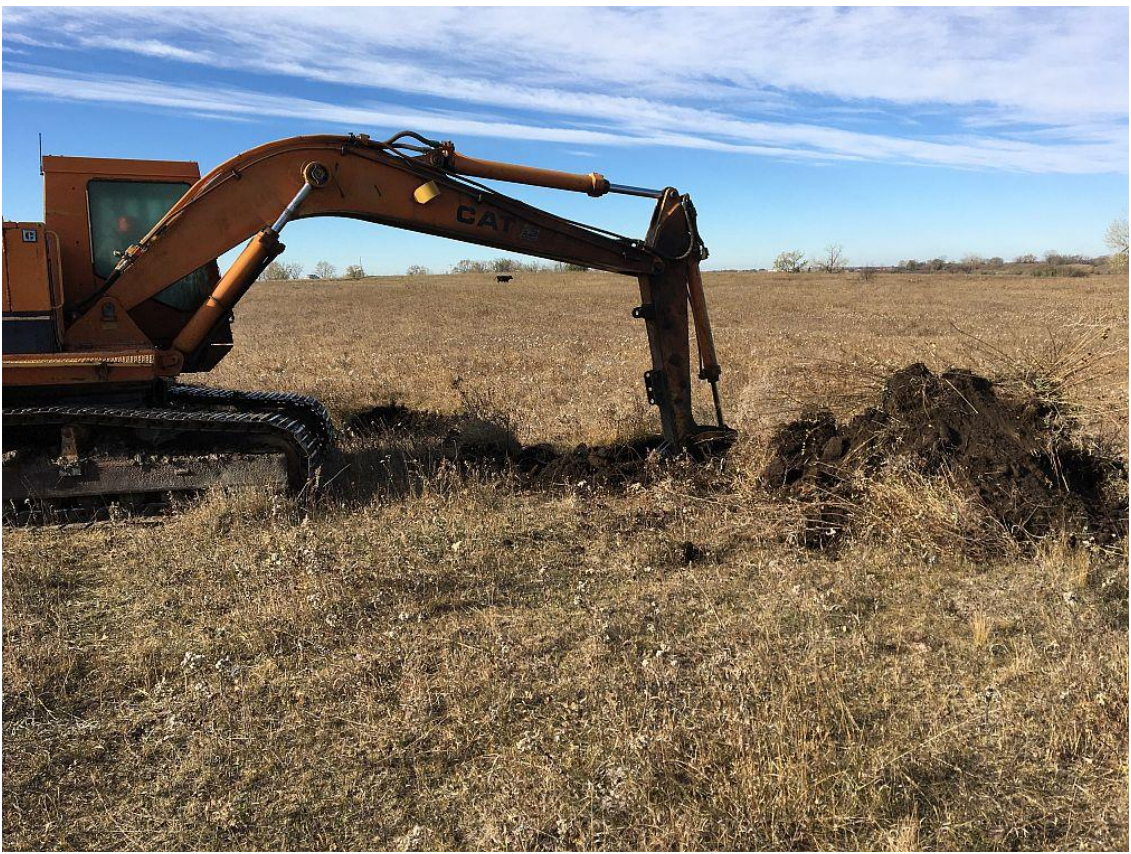
Approximately 41 sinkholes were filled on a pasture owned by Jim Krzmarzick about three miles southeast of Wilton. This shows an excavator saving topsoil from a dangerous sinkhole.
