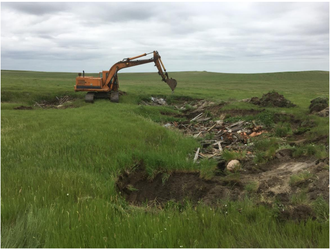
This shows a series of sinkholes at the Heil (Comet) site, owned by Rocky Ulrich and located about 2 miles southwest of Heil. Eighty sinkholes were filled on pastureland and cropland at this site. Inert waste had to be crushed and buried in many of them.
