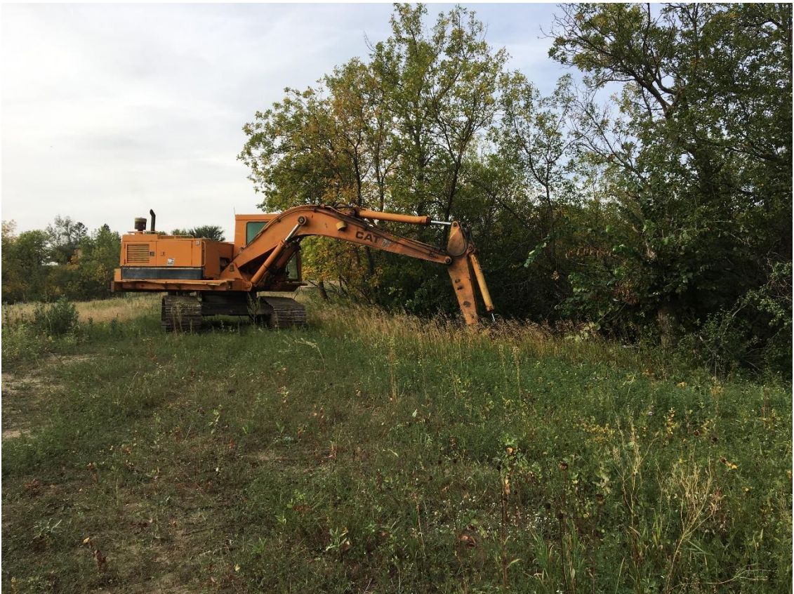
Two sinkholes were filled at this site on September 13. The approximate cost for this work was $1895. About 25 dangerous sinkholes have been filled near Richardton over the past ten years.
