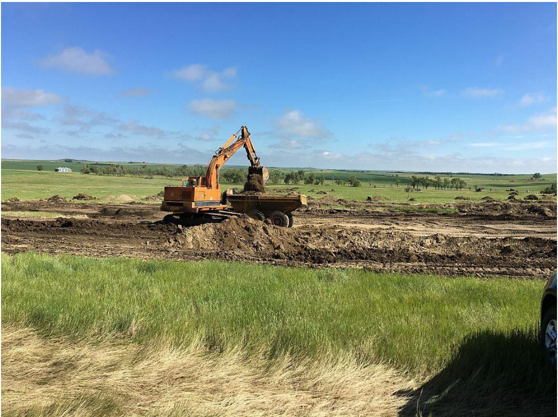
This shows a truck being loaded with fill dirt. The dirt piles in the background are topsoil which was removed from around the sinkholes. Work was conducted at this site between June 19 and July 9 and the contract cost for this work was $49,976.25.
