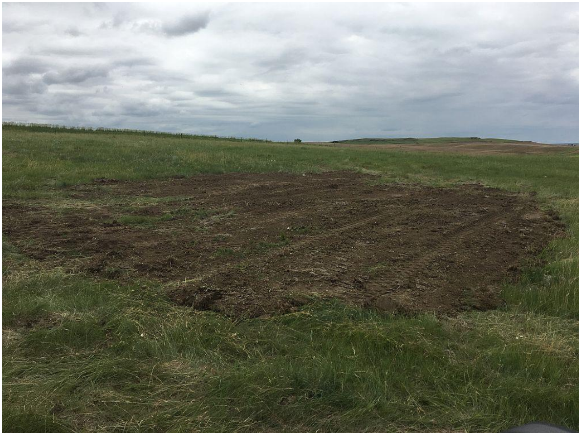
Eight sinkholes were filled at the New Leipzig site on June 18, 2018. This photo shows one that was filled, topsoiled, tilled and seeded to a seed mixture of native grasses. The contract cost for this work was $1696.25.
