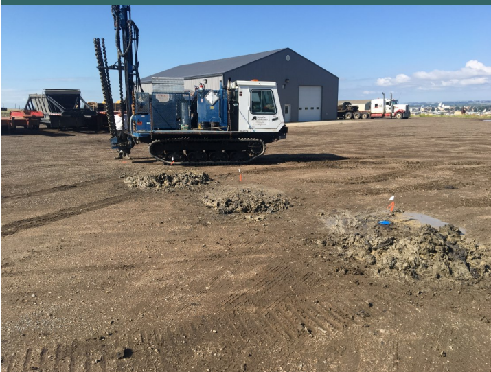
This drill rig ready to begin drilling a new hole. Piles of cuttings show the locations of recently drilled holes.
