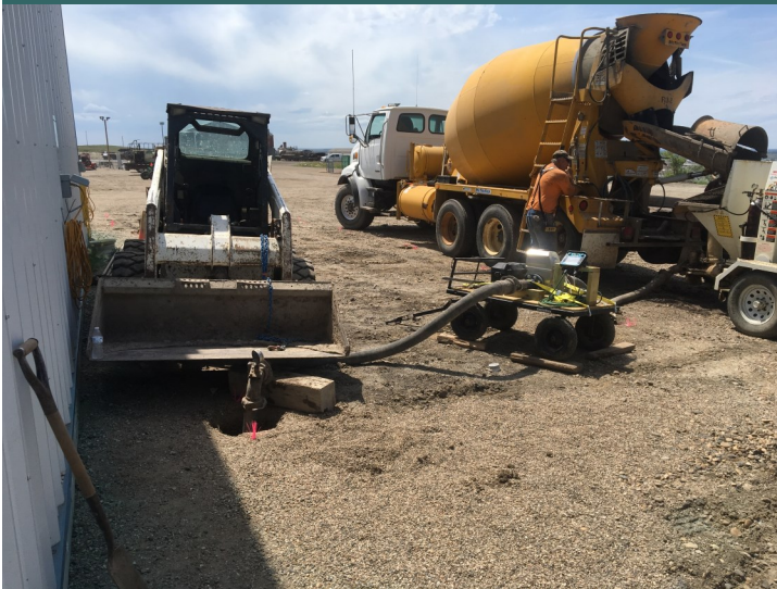
The grout runs through the meter to monitor the pressure. It then goes into the cased hole right next to a building.
