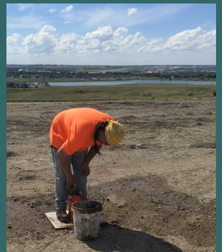
The material tester is doing a slump test on grout at Williston.
