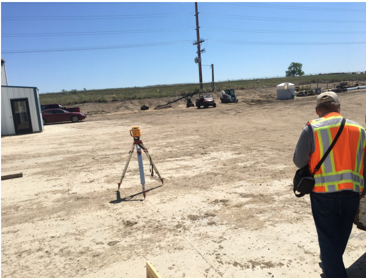
A laser level monitors ground movement near the Shift Services building during grout pumping. Inspector, James Thornburg, is on the right.
