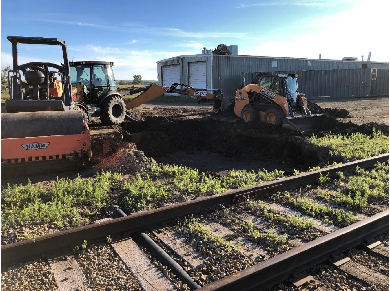
Figure 3: The sinkhole was over-excavated and is being filled and compacted. The landowner was concerned about the privately owned railroad track.
