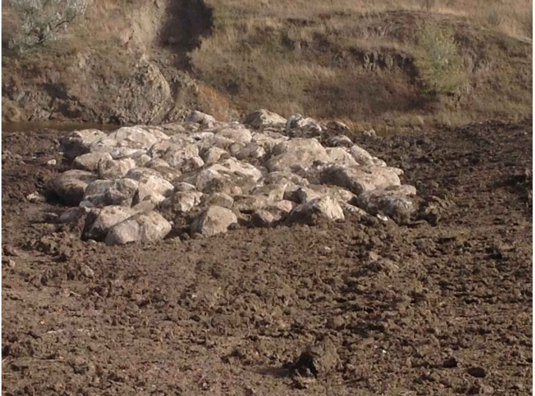
Rock Riprap Channel Established Downstream from Wetland Sump
