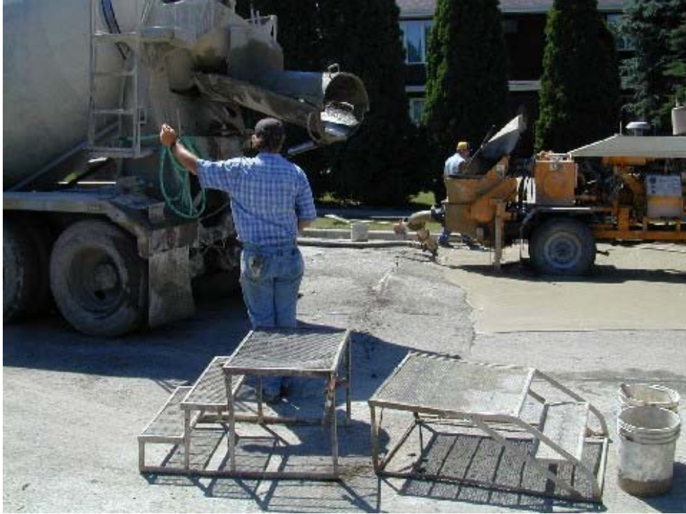
Figure 5: Surface lifting caused by pressurized grout remote backfilling on 1 st Ave. in Beulah.
