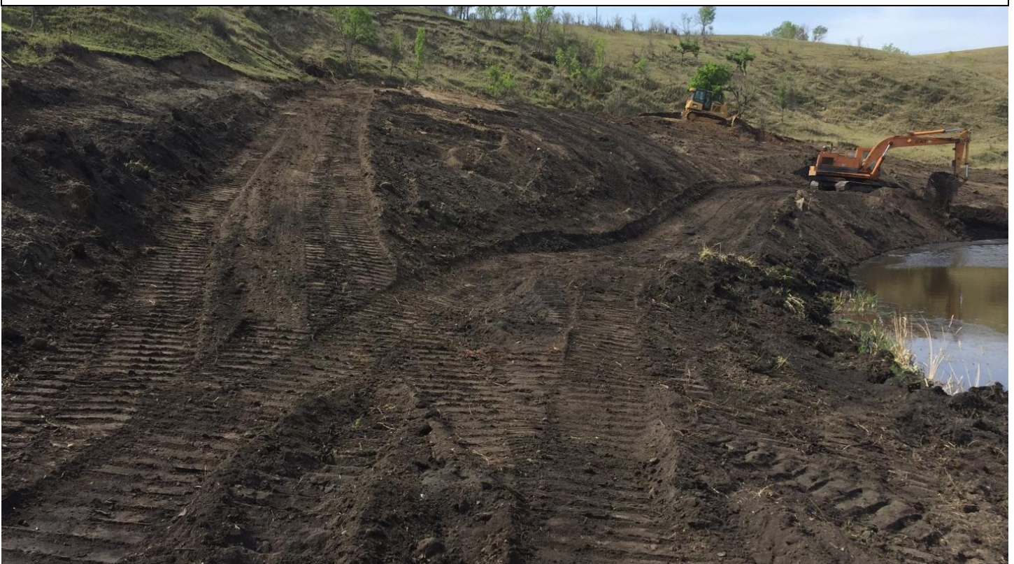
Below: Nearing completion, final mixing of coal refuse that hadn't been burnt yet by excavator while dozer pushes topsoil across area on June 5, 2015
