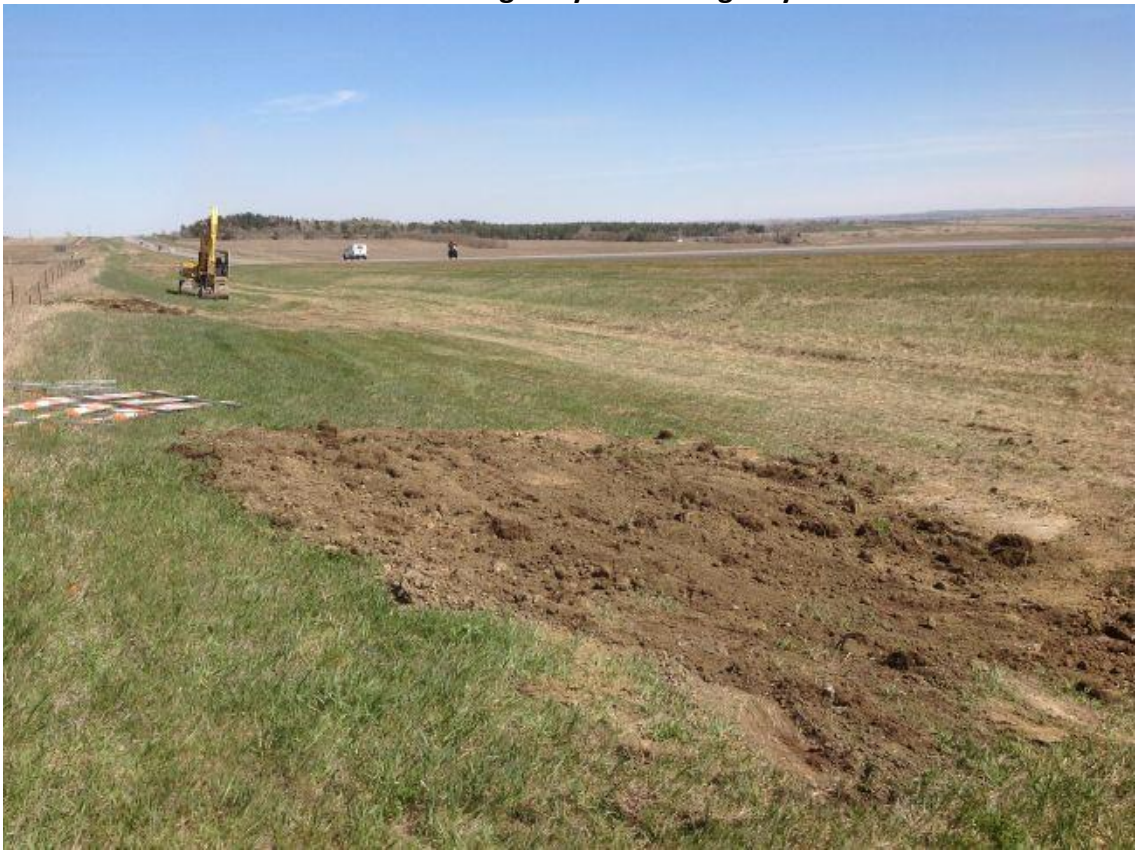
This photo shows the sinkholes on the ditch of Highway 200 on April 28 after they were filled and topsoil was respread.
