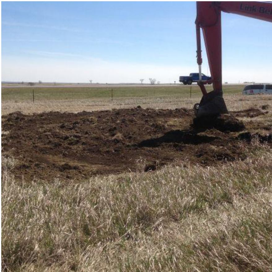
This photo shows the sinkhole with the fiber optic cables after it was filled and topsoil was being replaced. Five dangerous sinkholes were filled in this emergency project and the contract cost was $4945.
