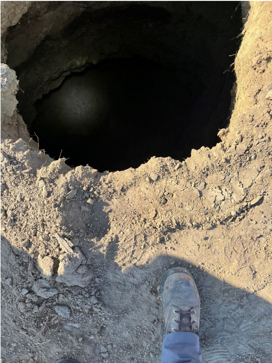
Figure 4: This sinkhole developed when heavy equipment was grading the highwall.
