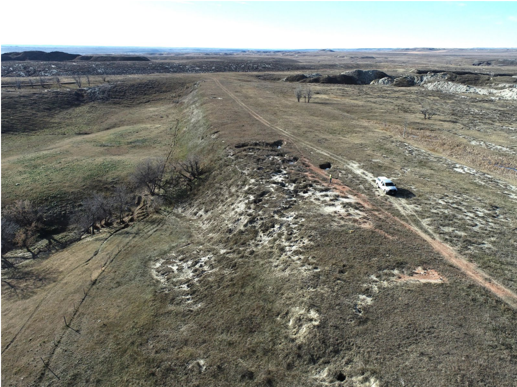
Figure 8: Slope stability area with subsidence features before reclamation.
