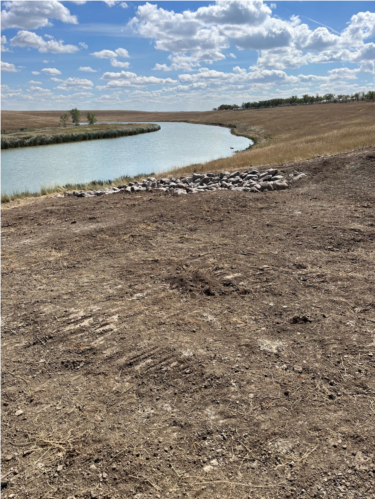
Figure 7: Three erosional gullies were graded and stabilized with rip rap in Section 36.
