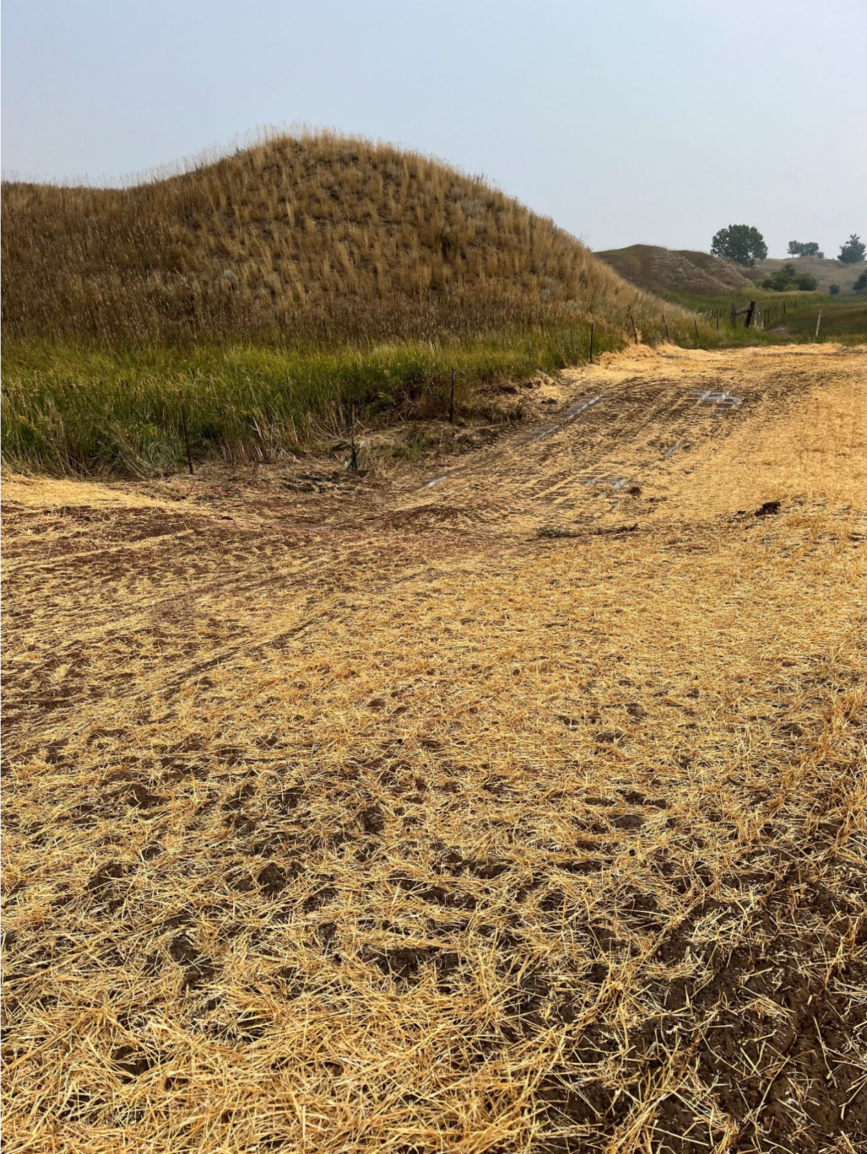
Figure 10: A flexible concrete mat was installed to replace a culvert and stabilize erosion.
